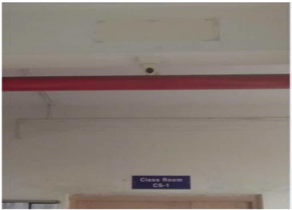
Camera on class room entrance
