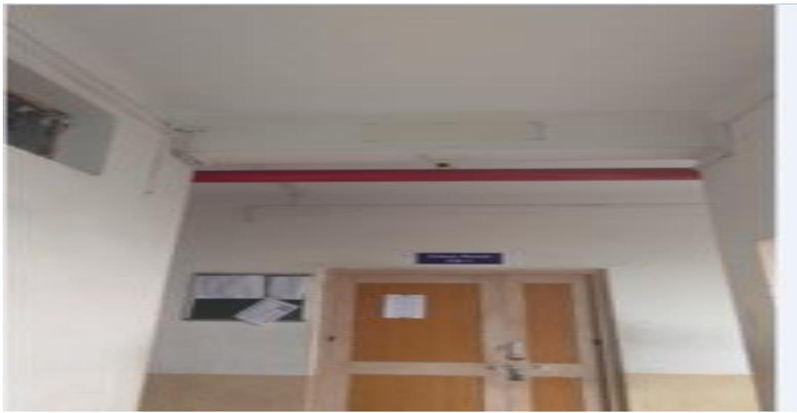
Camera on class room entrance
